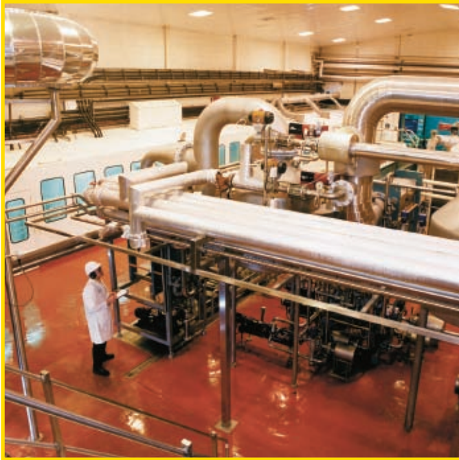
Investment in our low shear pumps at a yeast production facility has increased efficiency
