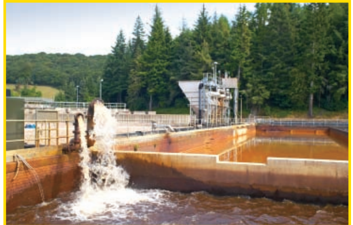
At a remote water treatment plant, a 2000:1 chemical flow range is required to balance pH levels
