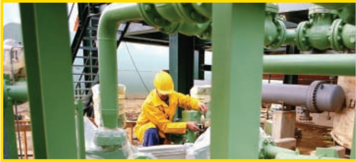
In an aggressive chemical recovery application, the pump paid for itself in less than 12 months
