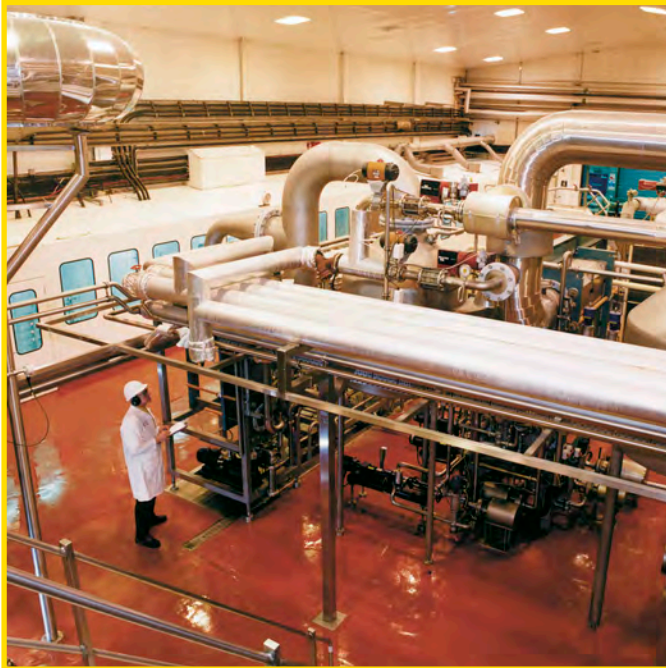
Investment in our low shear pumps at a yeast production facility has increased efficiency
