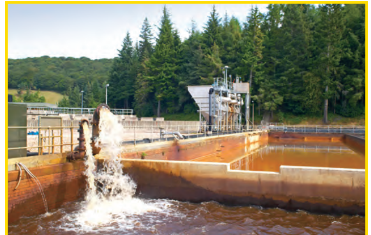
At a remote water treatment works, chemicals are metered to balance pH levels
