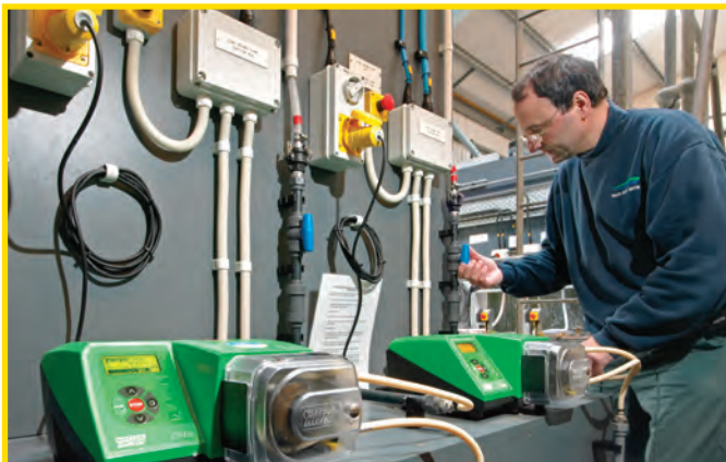
500 series pumps replaced troublesome diaphragm pumps for coagulant dosing
