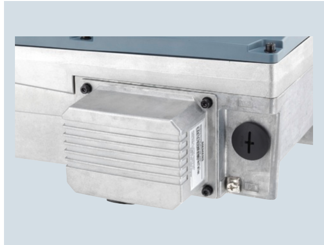
Fig. 9/23 24 V DC power supply, installed
