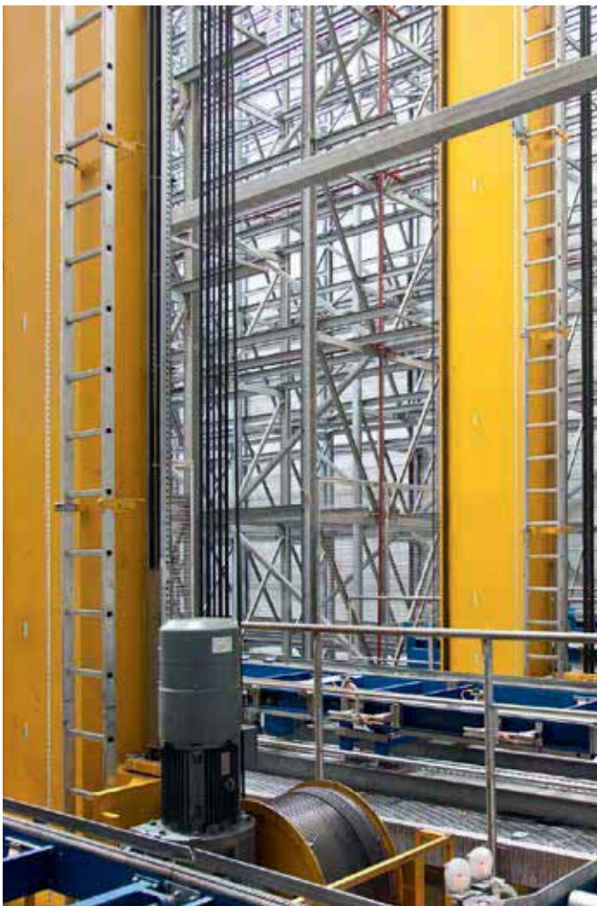
Storage/retrieval system (SRS)
