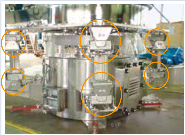
Gyratory screening machine installed on 8 pcs. AK-I 40 universal joints (joints made out of stainless steel)
