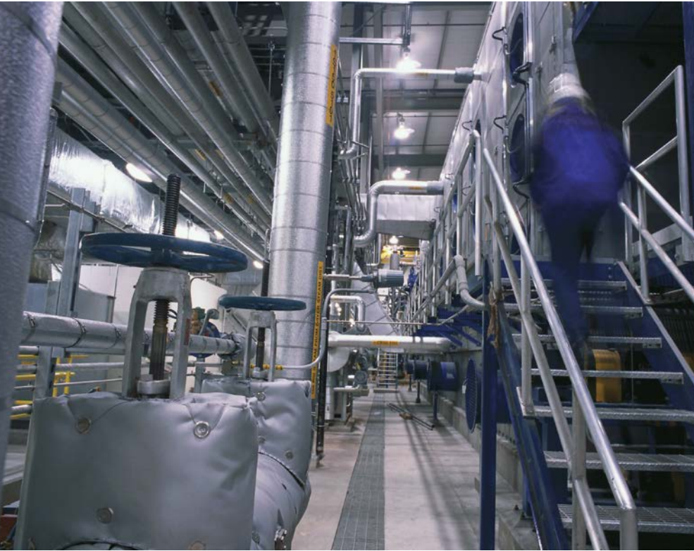
Plant control solutions
