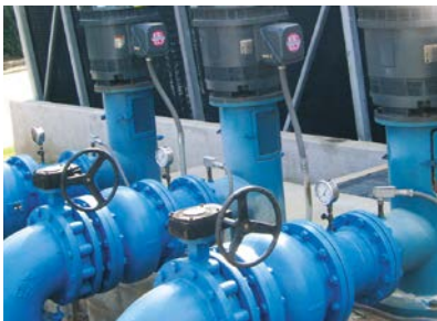
Complex processes involving liquids, pressures, temperatures can often need fast PID control algorithms.
