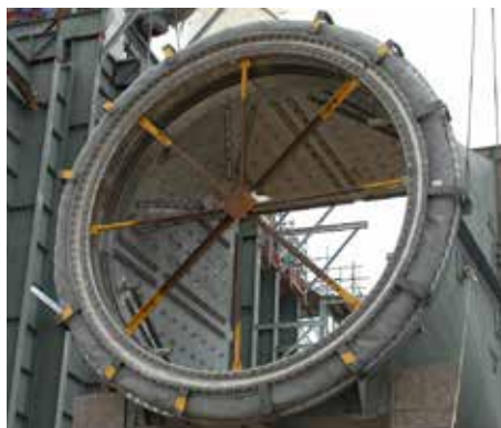
Installation of Combine-X on diffuser.
