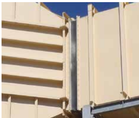
Acouseal installed in gas turbine air inlet.
