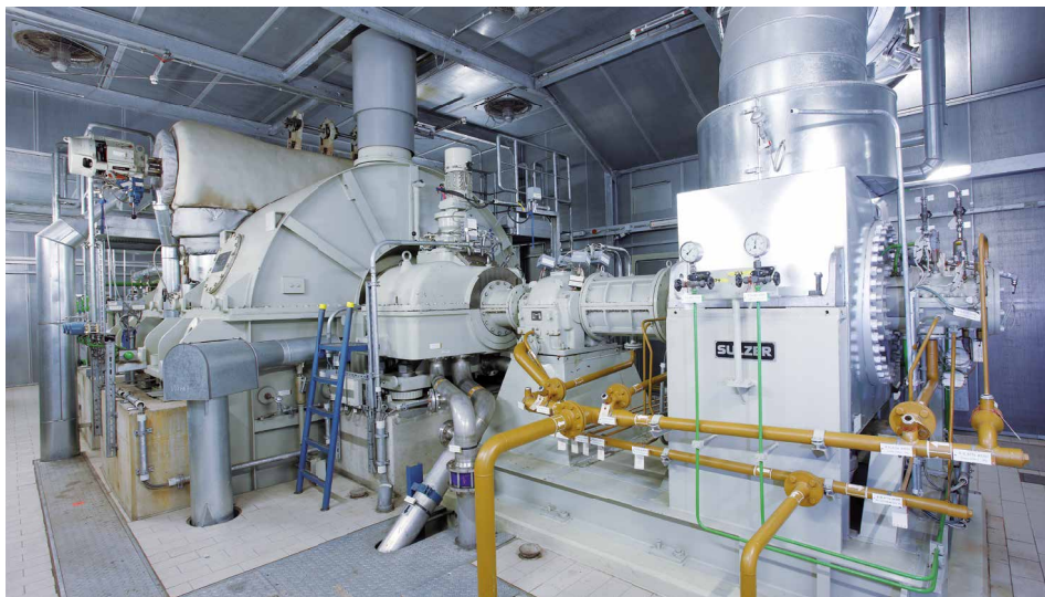
Steam turbine, lignite-fired power plant
