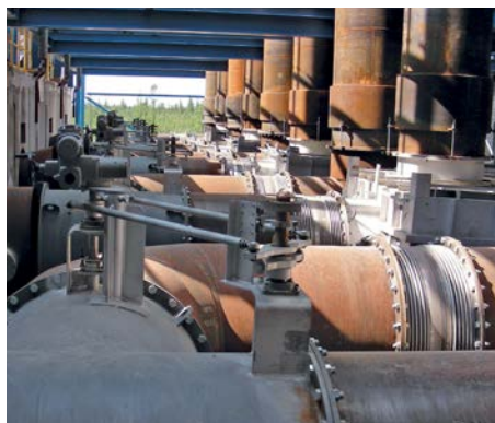
US-types installed in a flue gas system.
