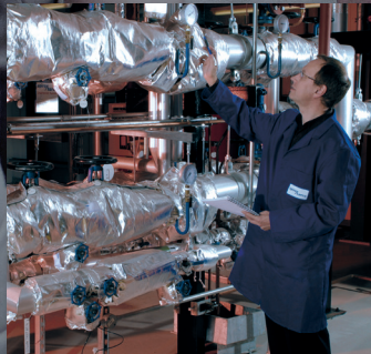
Ready assembled control systems
